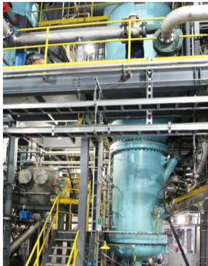
Figure 2: One of Genomatica's patents describes how to use syngas as a raw material, or feedstock, for the production of major chemicals. Shown here: plant producing syngas from municipal solid waste. Picture, courtesy of Enerkem.
